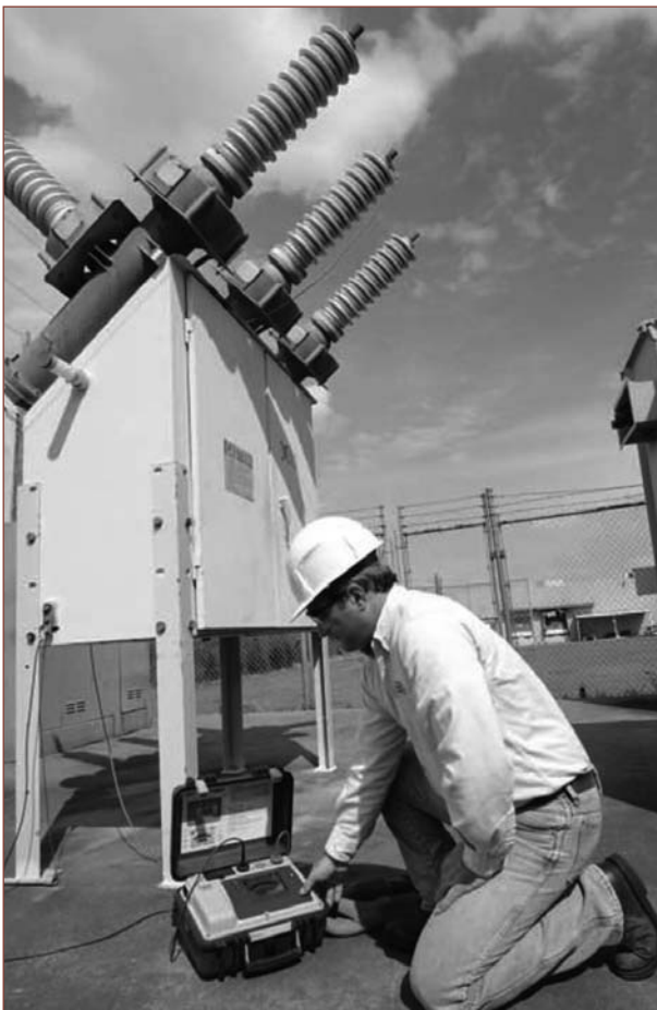
The MIT1020 in use at an industrial complex substation
