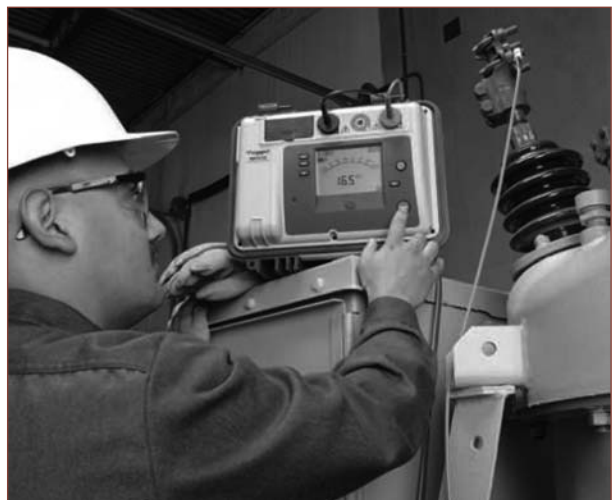
Delta wye transformer being testing with a MIT520
